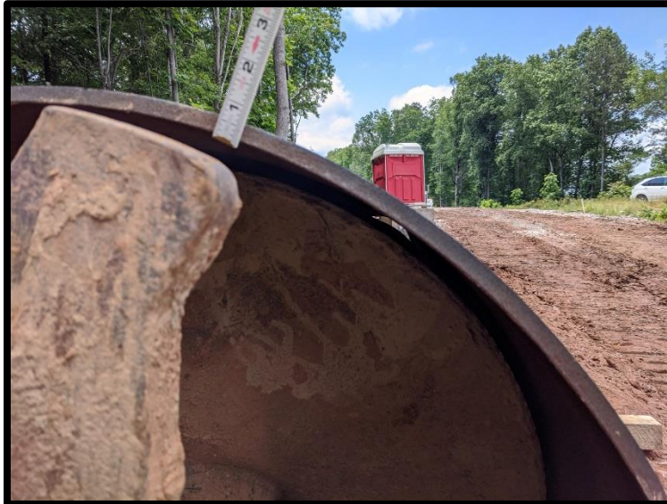
The image above illustrates the wall thickness of the steel casing pipe.
